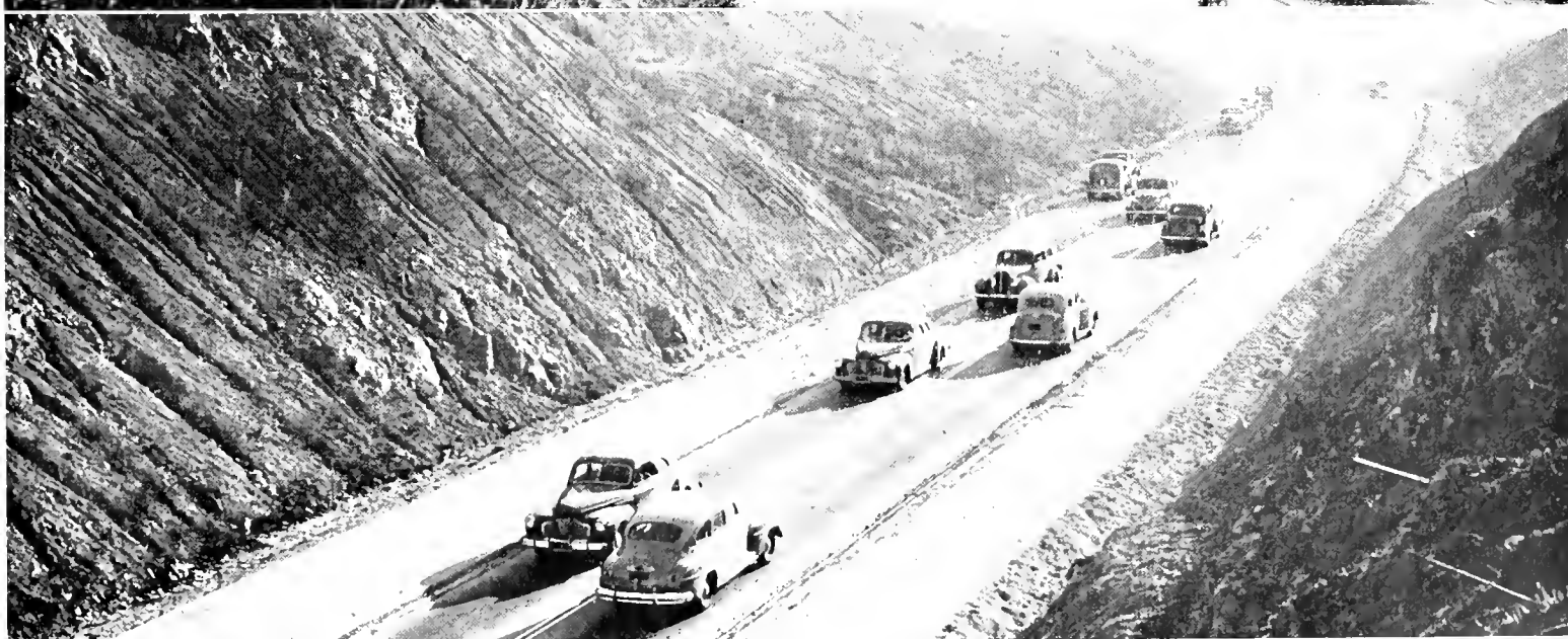
Adding extra lanes to 2-lane sections of American Canyon Cut-off (U. S. 40) to eliminate congestion on vertical curves through cuts.
